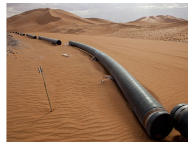
Pipeline construction in the Sahara desert. © Richard J Greenman / Alamy Stock Photo
